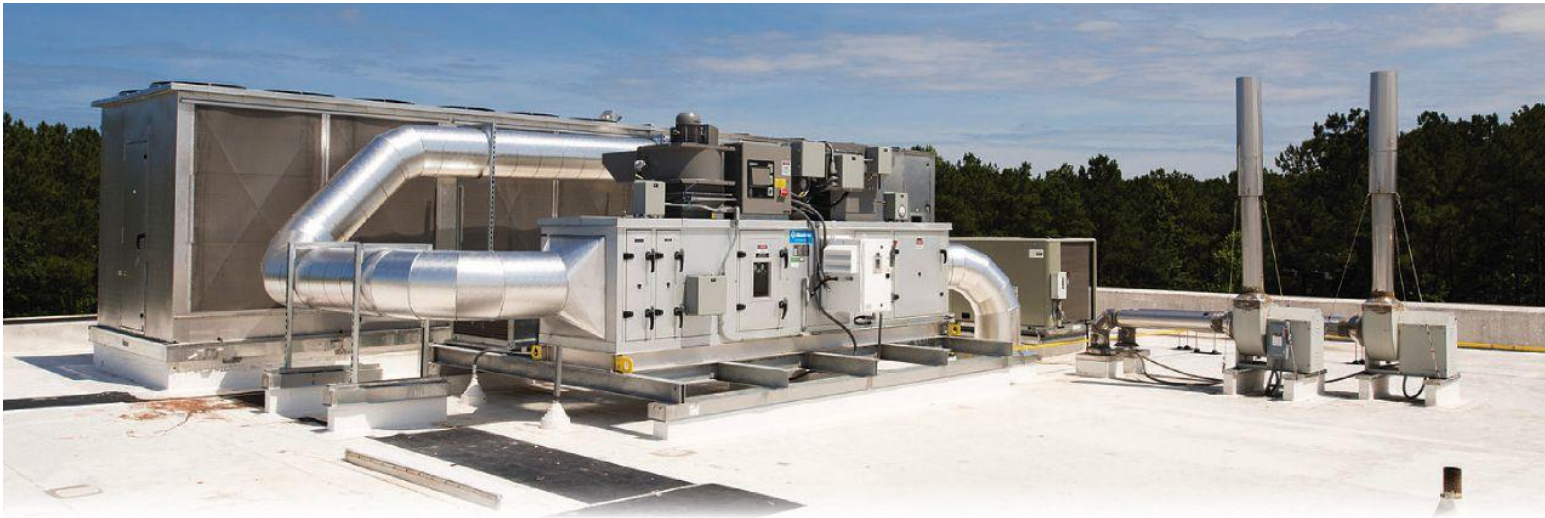
FIGURE 4: Tech center and lab mechanical, electrical and plumbing design and construction support services by CRB for a confidential client. Courtesy: CRB
