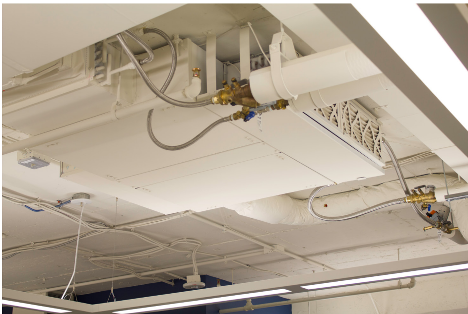
DOAS Terminal Unit in Exposed Ceiling | 1325 G Street NW | Washington, DC
